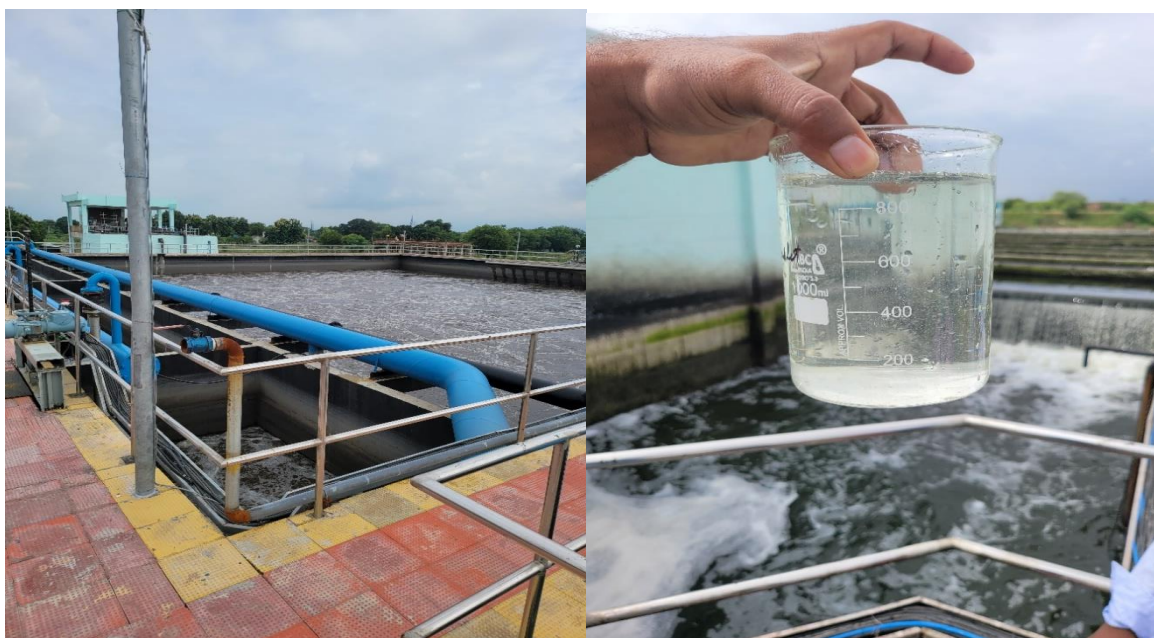
Figures 4.11 A & B: 50 MLD Ramana STP and Treated sewage
