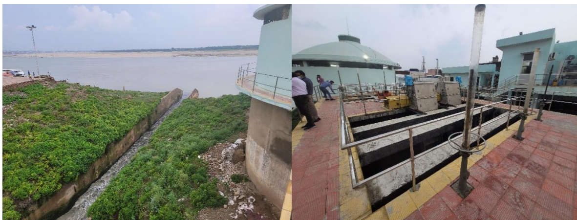
Figures 4.10 A & B: Assi River joining River Ganga and 50 MLD Nagwa Pumping Station
