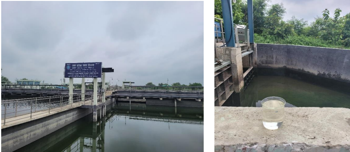
Figure 4.6: 120 MLD STP at Goitaha for catering flow of trans Varuna Region
