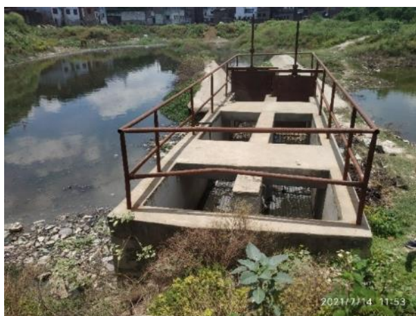
P 23: Ponding Near Nakhi Drain
