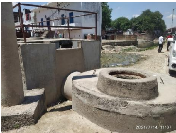
P 25: Narokhar drain (Tapped)
