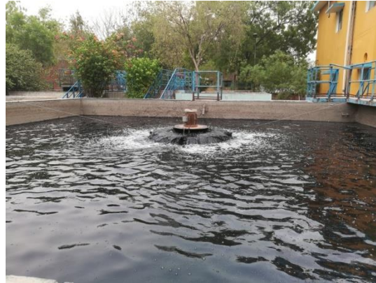
Figure 12: Poor mixing in equalization tank
