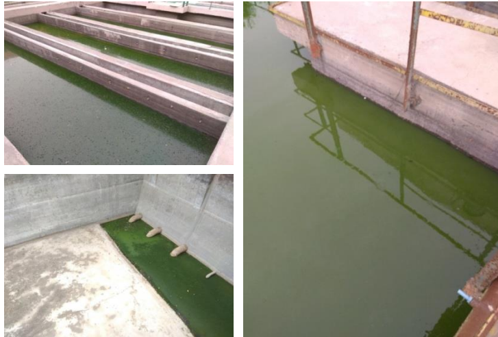
Figure 17: Non-operational CETP at Okhla
