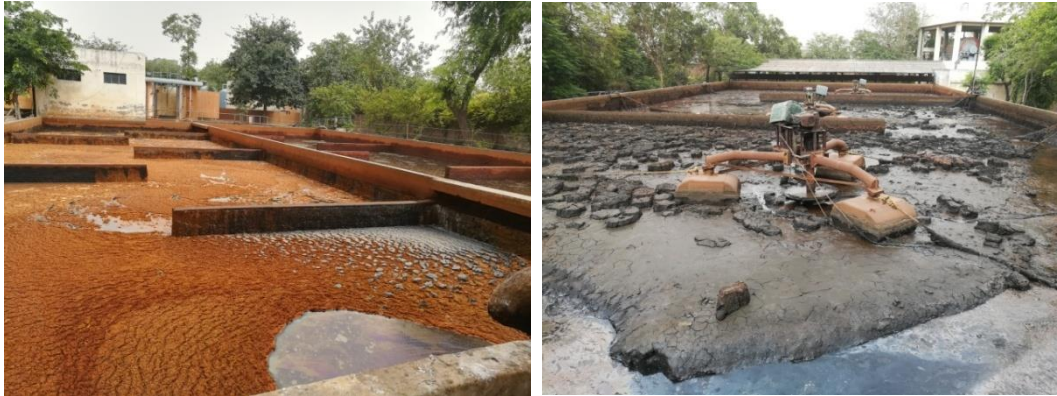
Figure11: Pre-Chlorination Tank (left) and flocculation chamber (right)
