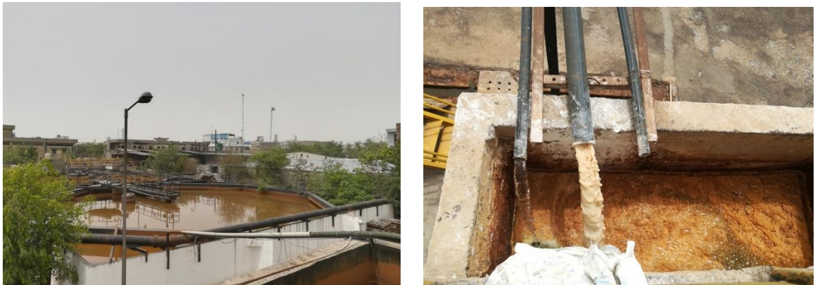
Figure 9: Equalization Tank (left) & inadequate dosing arrangement (right)
