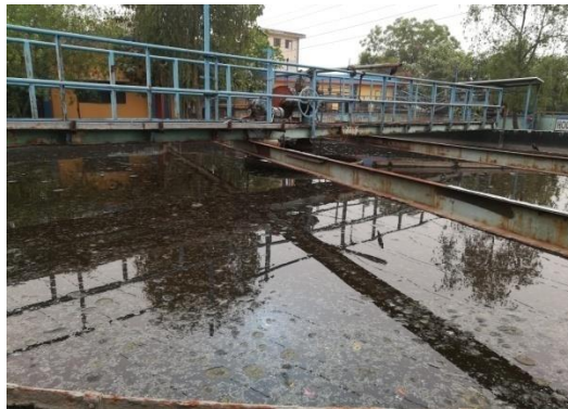
Figure13: Poorly managed Clariflocculator
