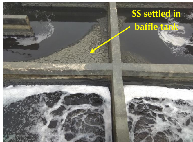
Figure16: SS settled in Baffle tank
