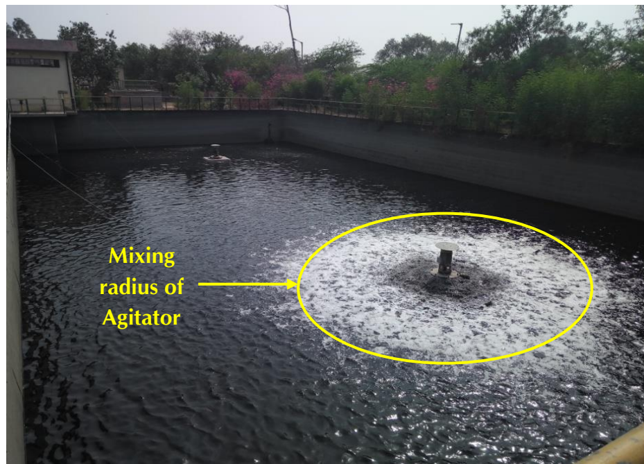
Figure 5: Inadequate mixing at Equalization Basin
