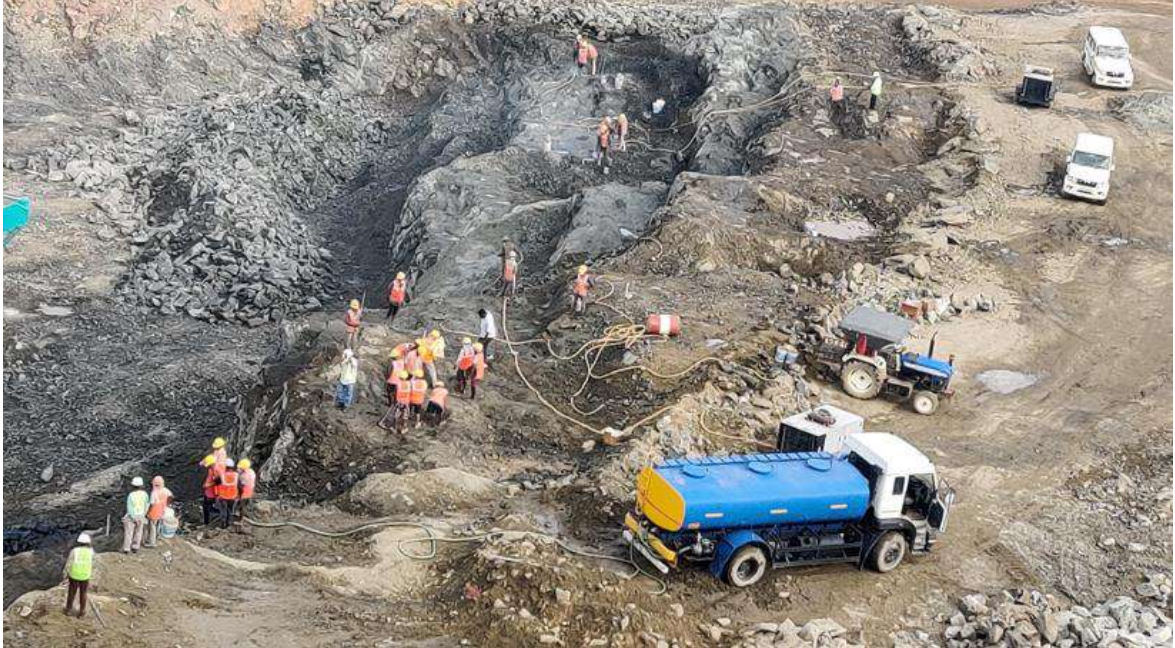
Plate 5.4.5. Drilling of blast holes using Jackhammer drill machine at Parackal Stone Quarry
