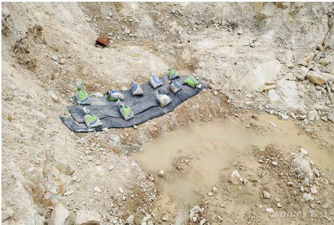
Plate 5.2.6. View of muffling arrangement made at granite building stone quarry of Muhammad Roshen
