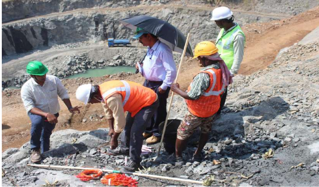
Plate 5.7.4. Charging of blast holes at Granite (Building Stone) Quarry, Palakkad District of Kerala State
