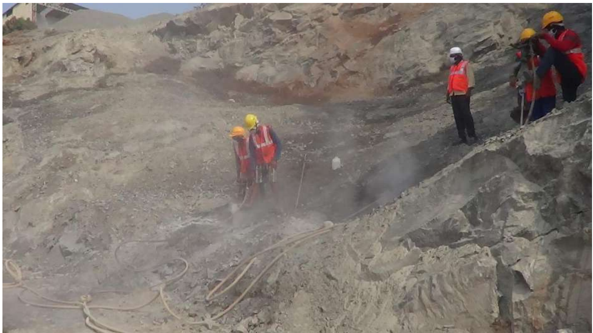
Plate 5.7.3. Drilling of blast holes using Handheld Jackhammer drill machine at Granite (Building Stone) Quarry of M/S Penta Granites, Palakkad District of Kerala State
