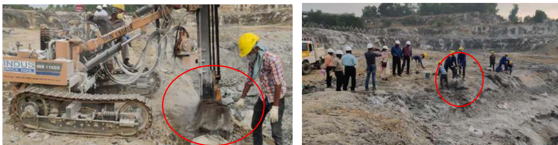
Plate 5.3.3. View of crawler-mounted pneumatic drill machine with wet gunny sacks and Jackhammer drill machine being used for drilling of holes
