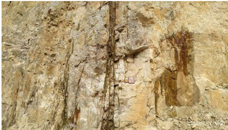
Plate 5.2.2. View of closely spacing joints dipping towards East
