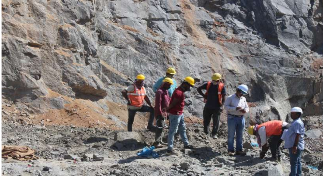
Plate 5.8.4. Charging of holes at Granite Stone Quarry owned by Sudheesh A. T., Wayanad District of Kerala State
