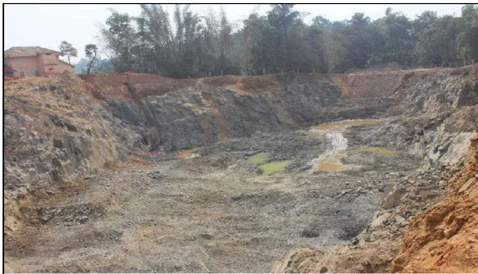
Plate 5.8.1. The overview of Granite Stone Quarry owned by Sudheesh A. T., Wayanad District of Kerala State
