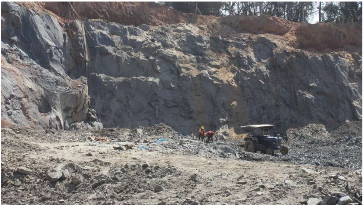
Plate 5.8.3. Drilling of blast holes using Handheld Jackhammer drill machine at Granite Stone Quarry owned by Sudheesh A. T., Wayanad District of Kerala State
