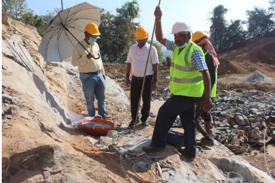
Plate 5.9.4. Charging of holes at Granite Building Stone Quarry owned by P. M. Abdul Rahaman, Kasargod District of Kerala State
