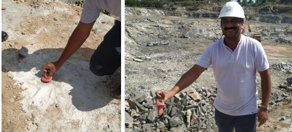
Plate 5.3.4. View of hole cap for inadvertent filling of holes and to maintain correct depth of hole prior to putting explosive into the holes
