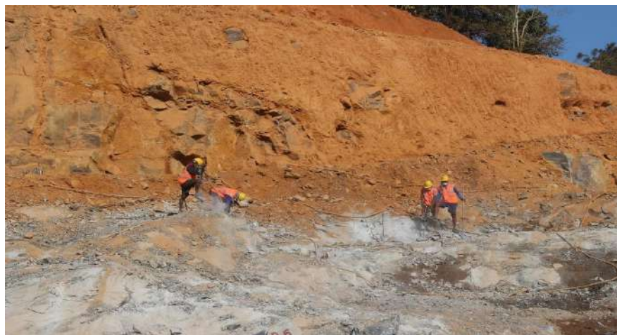
Plate 5.9.3. Drilling of blast holes using Handheld Jackhammer drill machine at Granite Building Stone Quarry owned by P. M. Abdul Rahaman, Kasargod District of Kerala State
