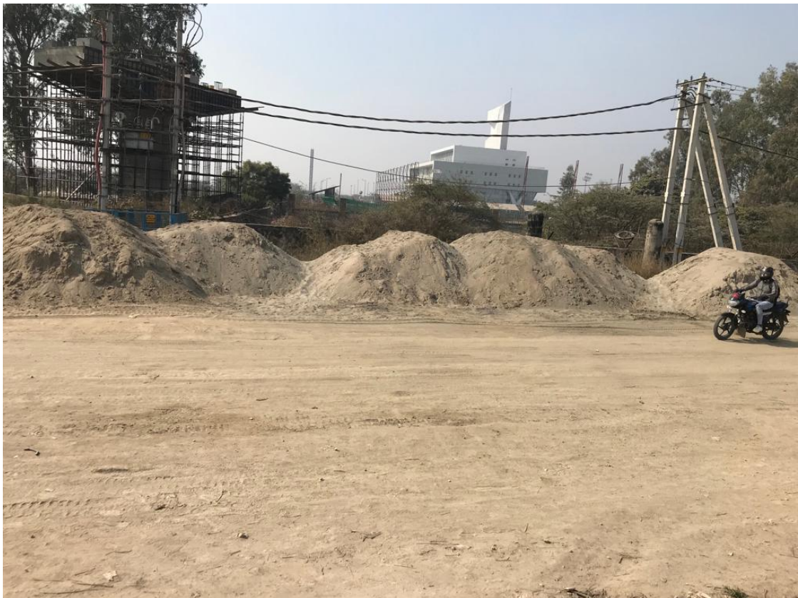
Photograph 4: Soil and sand kept uncovered on the Part of NHAI works adjoining to the NH-44.
