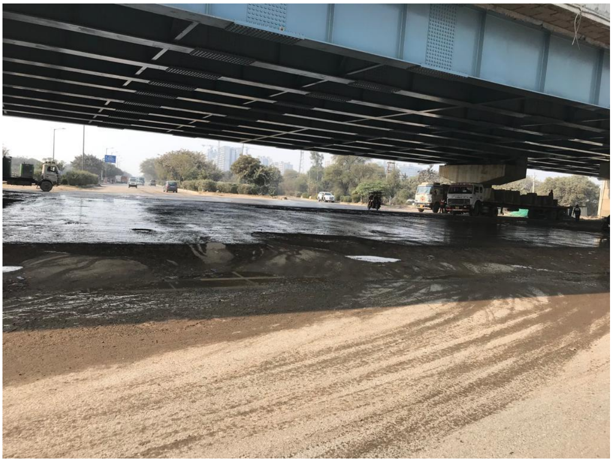
Photograph 5: Sprinkling being carried out on the Part of NHA I works adjoining to the NH-44.
