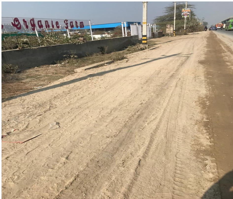
Photograph 6: Loose soil found on the parts of the stretch under reference.
