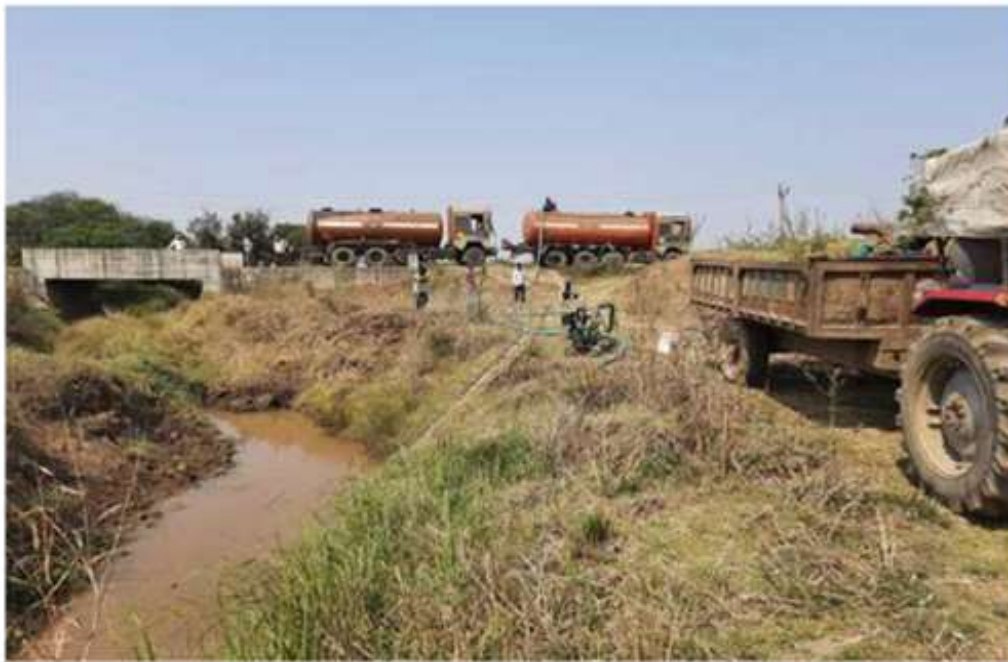
Wastewater lifting from Gumanpura village
