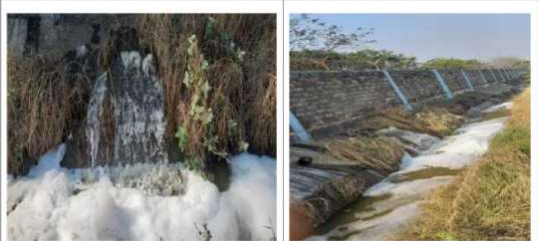
Contaminated water is coming out from the boundary wall of the unit at north side of unit area and going into GIDC storm water drain outside the unit
