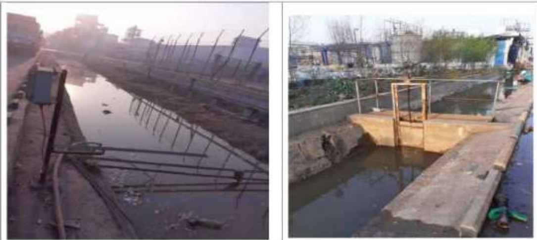
Contaminated water is observed accumulated in storm water drain within unit premises
