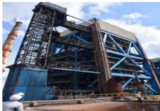
Figure 2 Steel structure supporting Boiler
