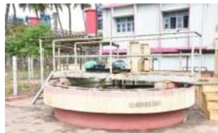
Figure 7 STP - Clarifier tank
