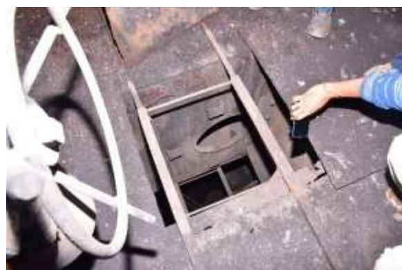
Figure 5 Opening at 15 ML girder, where smoldering was found
