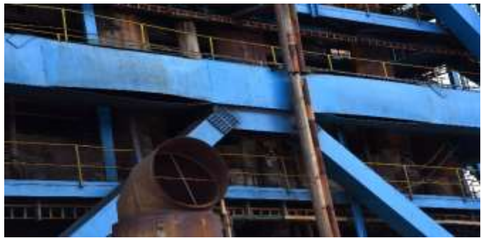
Figure 6 Damage to the girder
