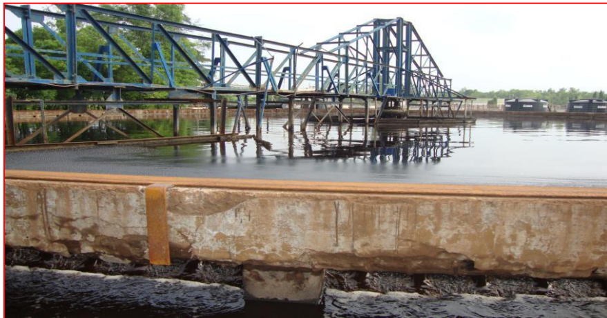
Photo-2 Primary Clarifier
