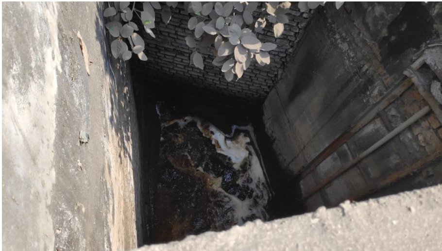
Photo-7 Treated effluent discharge chamber before discharge point
